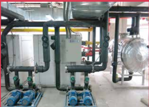
Heat pump; Water to water 200 kW x 2 set; 100 kW x 2 set Virgin Active.
