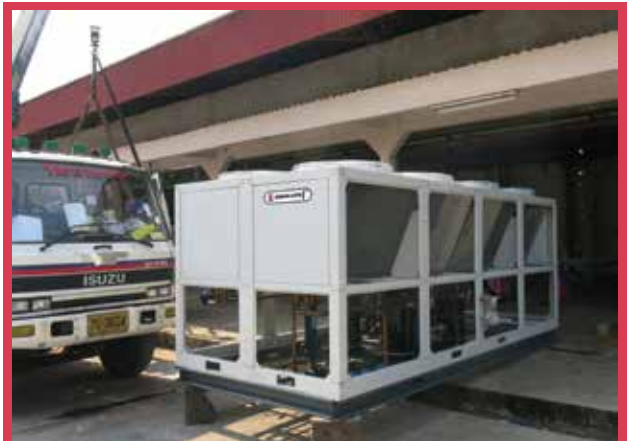
Air Cooled Chiller 60RT Air cooled chiller for 4 C coconut water. Coconut factory; Prachubkirikun
