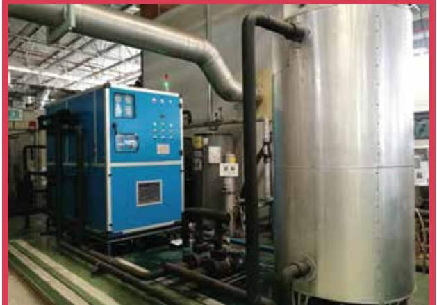
Heat pump; Water to water 210 kW x 1 set with hot water tank AGC Automotive.
