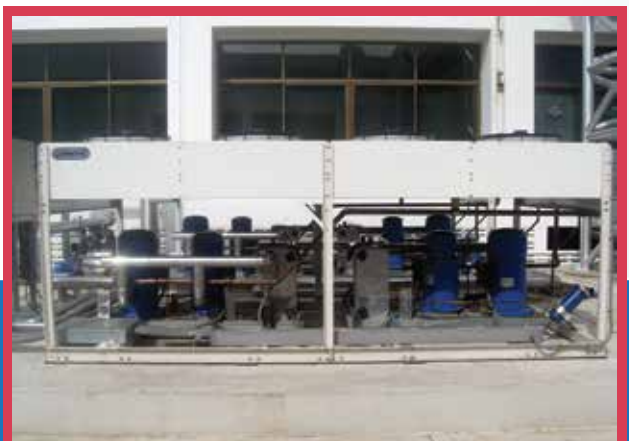
Air Cooled Chiller 60RT Air cooled chiller. Wangnoi Beverage.
