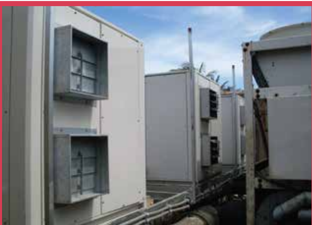
Heat pump; Air to water 45 kW x 3 set; replacement old system. Centara Grand Samui.
